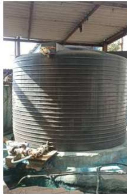
Spent acid storage tank
